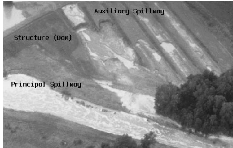
Fig. 3. Spillway erosion. (Image courtesy USDA)
